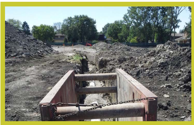
Storm sewer work can be messy and dusty. The Village and Contractor will work hard to keep everything clean.
