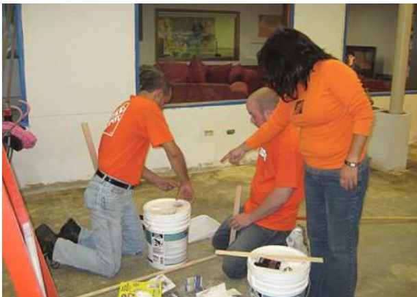
The expansion of the Niles Teen Center was mostly completed June 11 after several days of work from more than a dozen volunteers from Home Depot.
